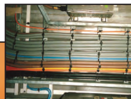
Marine Cable Bundling
